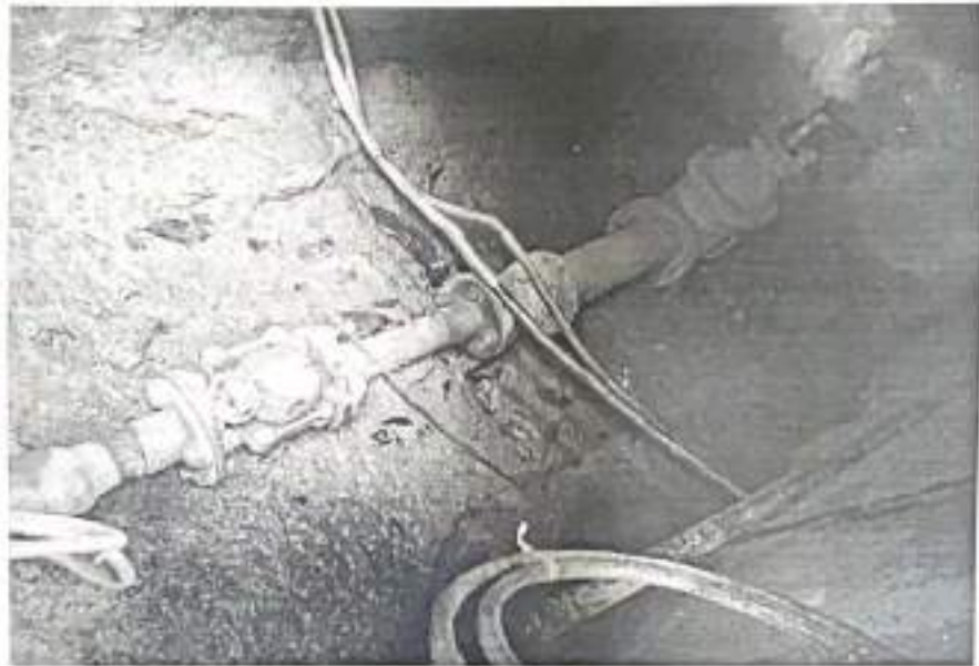
Figure 4-15: Water flow meter installed in the campus
