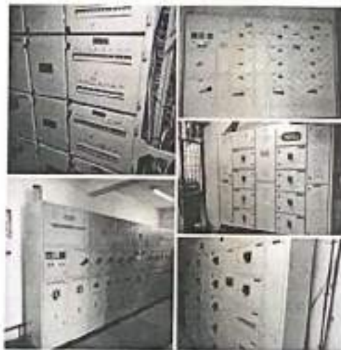
Figure 5-5: Electrical distribution panels in various blocks
