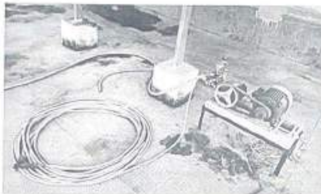
Figure 5-10 Pressurized water cleaning for SRTPV systems
