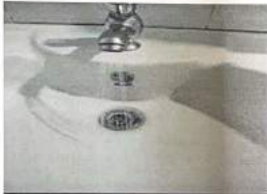
Figure 4-17: Low flow taps installed in the college
