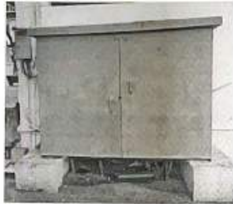
Figure 5-4: Feeder Pillar near NSB block
