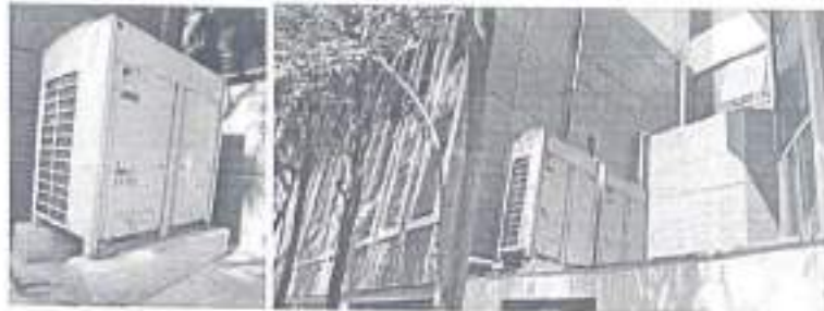
Figure 5-14: VRV Air Conditioning Unit
