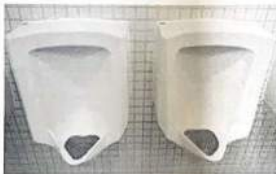
Figure 4-18: Water less urinals installed in the college
