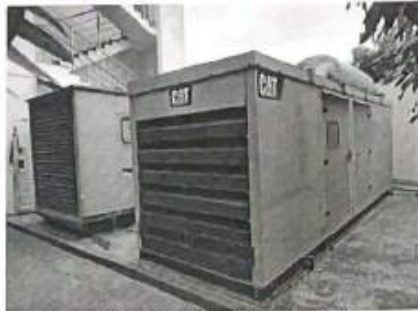
Figure 5-6: Diesel Generator (DG) sets
