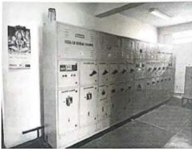
Figure 5-2: Electrical panel Room
