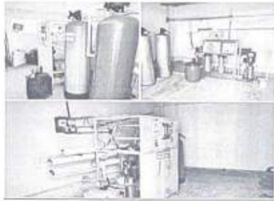
Figure 4-5: RO water treatment plant in the campus
