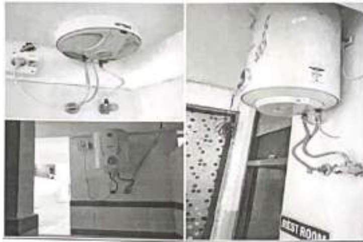
Figure 4-8: Electrical water heaters installed in hostels
