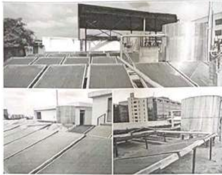
Figure 4-7: Solar water heater installed in the campus
