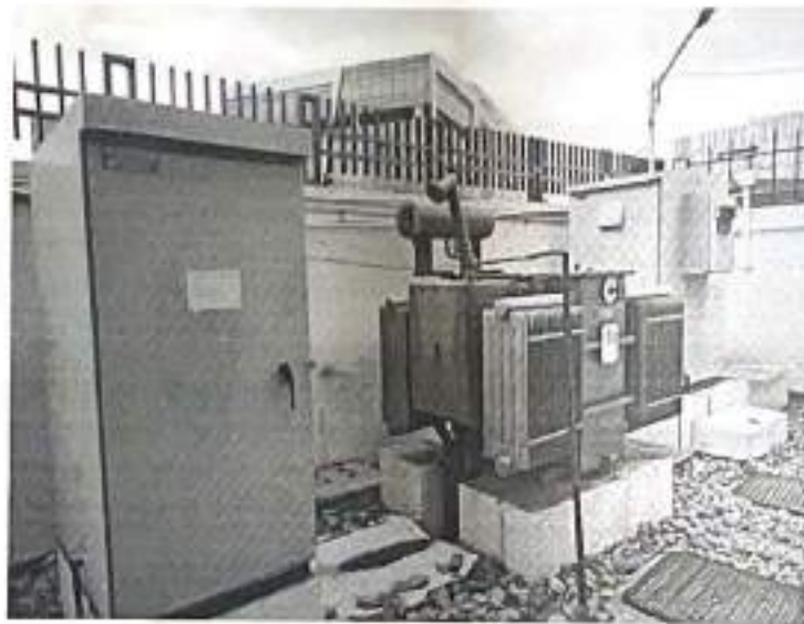
Figure 5-1: Transformer unit Installed in the campus
