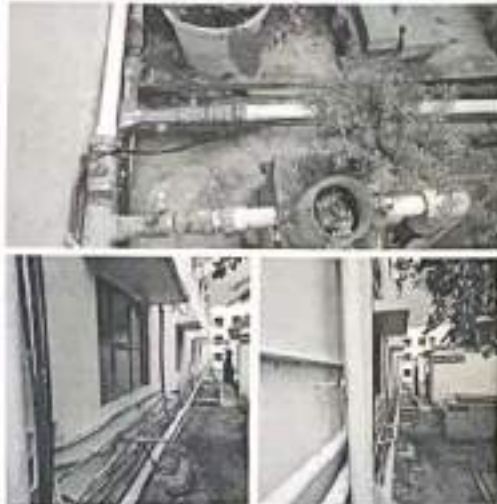
Figure 4-16: Dual water piping system installed in the campus
