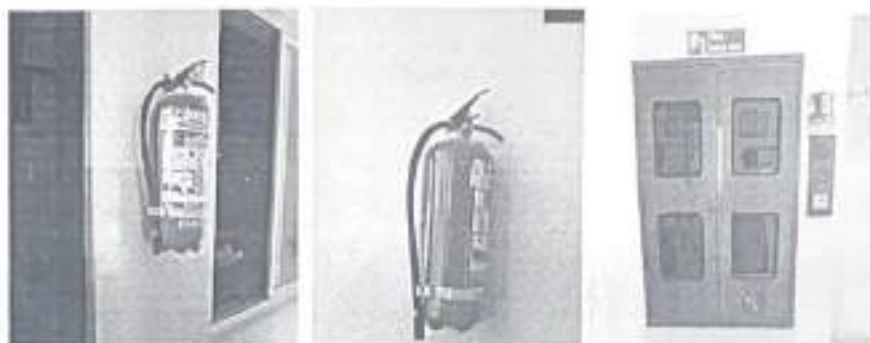
Figure 3-2: Fire Extinguisher and Fire hydrant system
