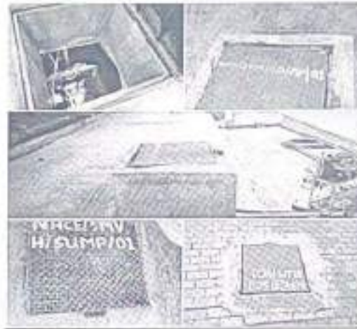
Figure 4-2: Sumps in the campus
