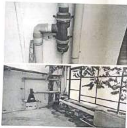
Figure 4-11: Rain water harvesting system in the campus
