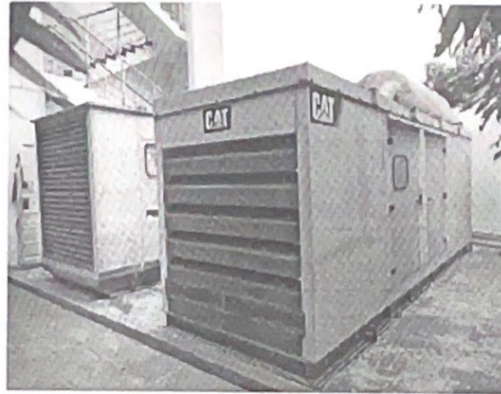
Diesel Generator (DG) sets
