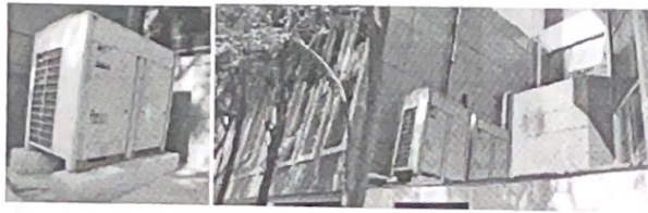
VRV Air Conditioning Unit
