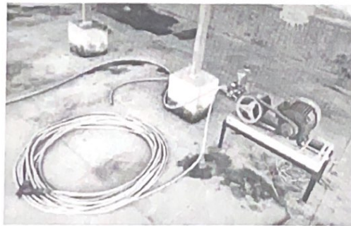
Pressurized water cleaning for SRTPV systems
