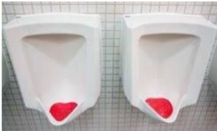
Figure 4-18: Water less urinals installed in the college
