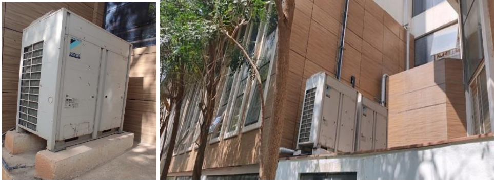
Figure 5-14: VRV Air Conditioning Unit
