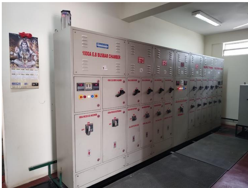
Figure 5-2: Electrical panel Room
