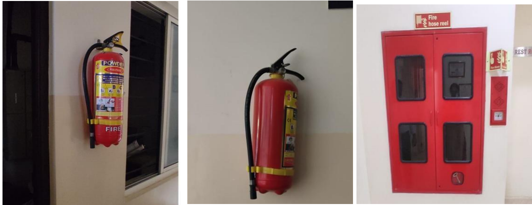
Figure 3-2: Fire Extinguisher and Fire hydrant system
