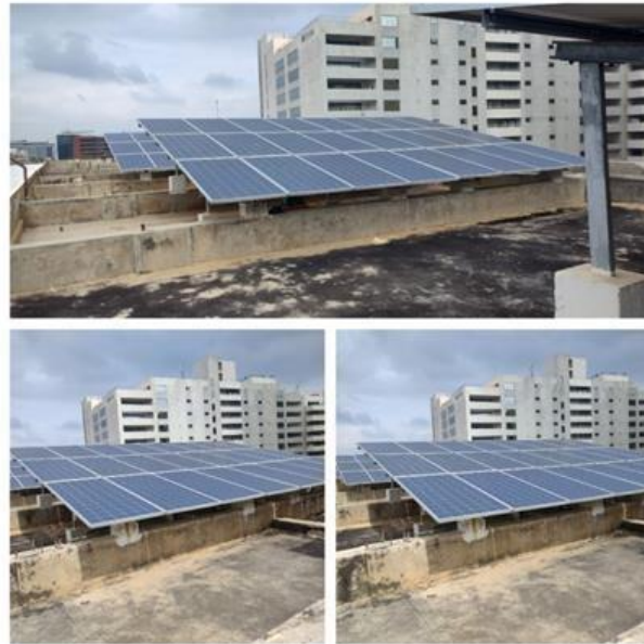
Figure 5-8: Solar rooftop PV system installed in SVP block
