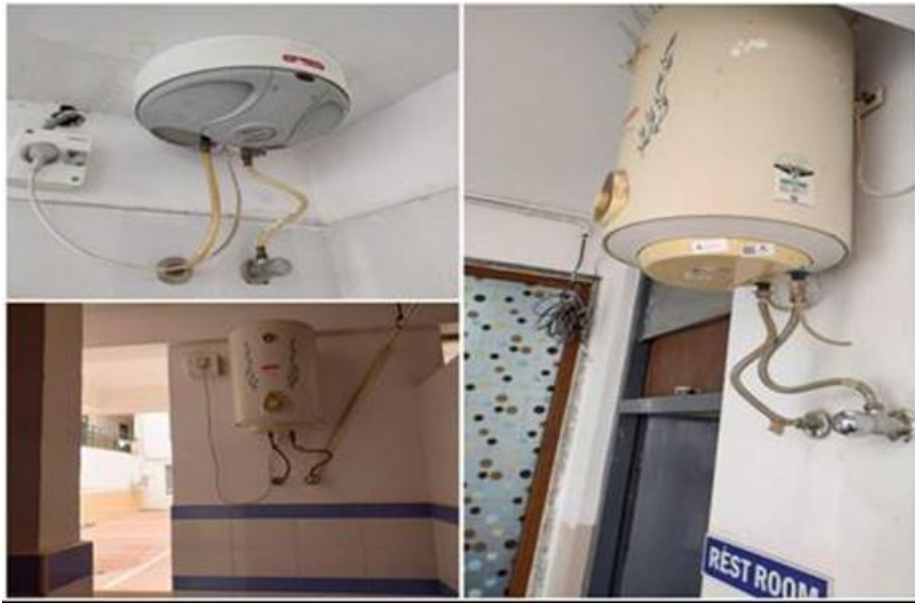
Figure 4-8: Electrical water heaters installed in hostels
