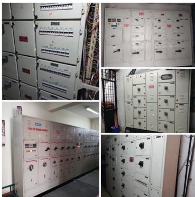
Figure 5-5: Electrical distribution panels in various blocks
