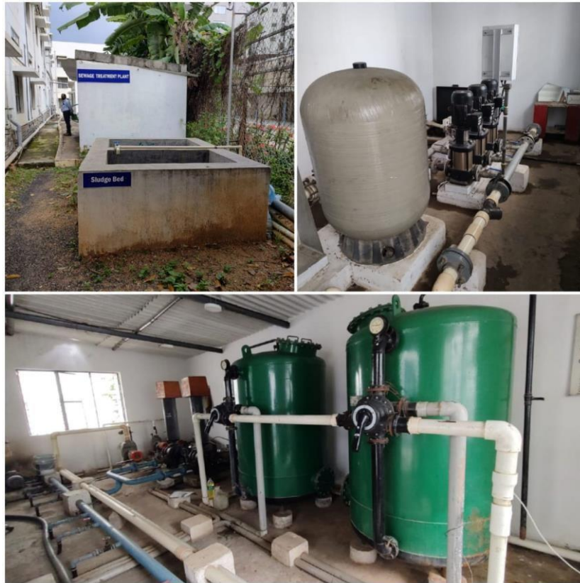
Figure 4-12: Sewage Treatment Plant
