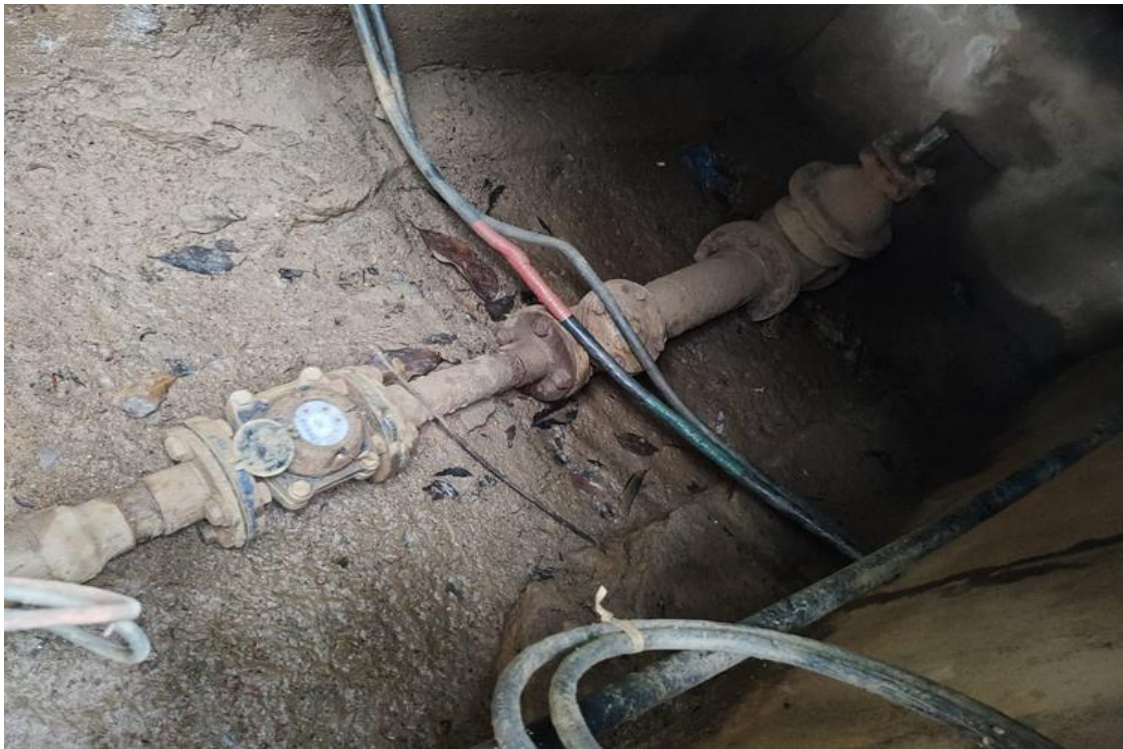
Figure 4-15: Water flow meter installed in the campus
