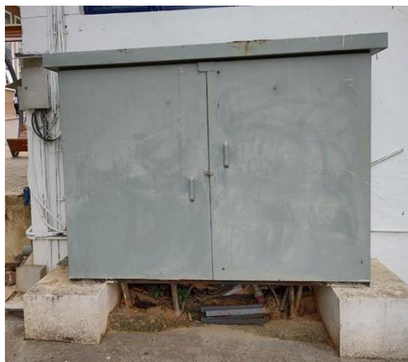
Figure 5-4: Feeder Pillar near NSB block
