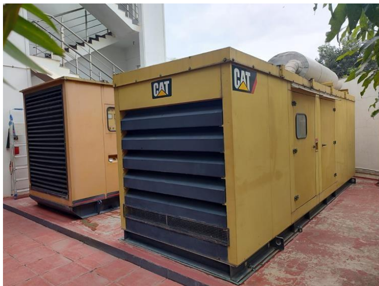
Figure 5-6: Diesel Generator (DG) sets
