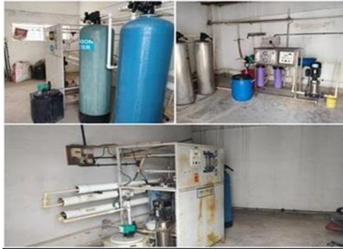
Figure 4-5: RO water treatment plant in the campus
