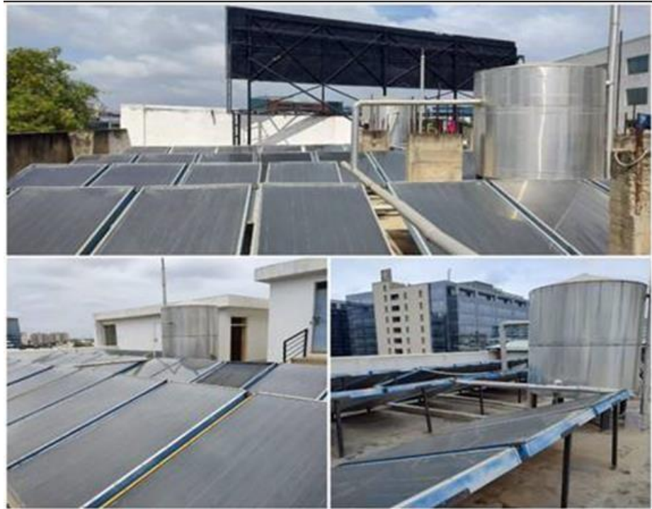
Figure 4-7: Solar water heater installed in the campus
