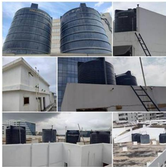
Figure 4-3: Overhead tanks in the campus
