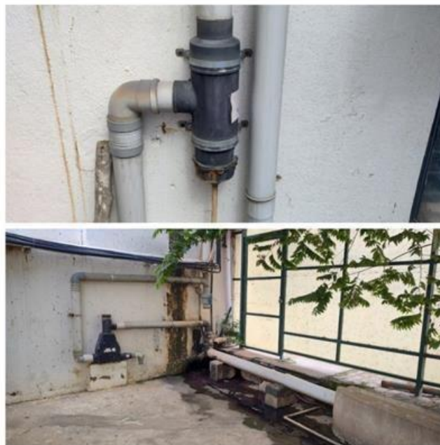
Figure 4-11: Rain water harvesting system in the campus
