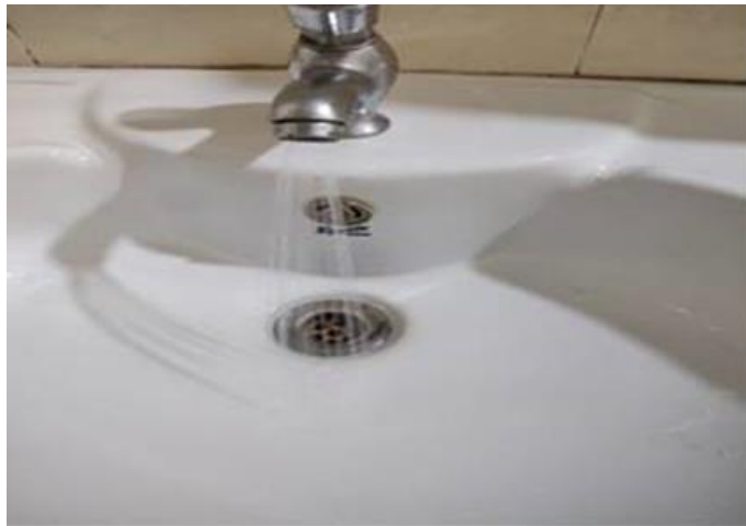
Figure 4-17: Low flow taps installed in the college
