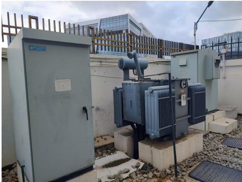
Figure 5-1: Transformer unit Installed in the campus
