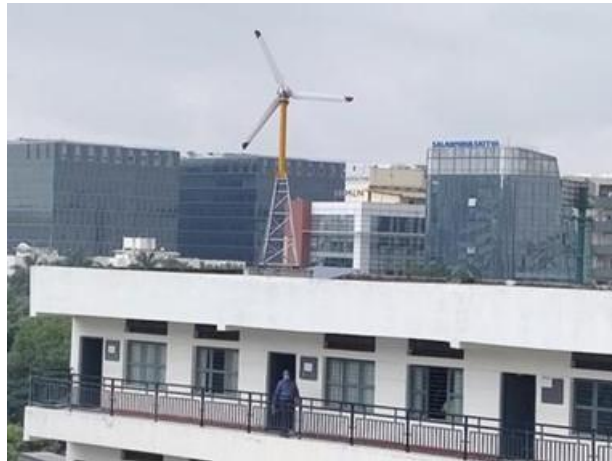
Figure 5-18: Micro wind mill installed in SVP block
