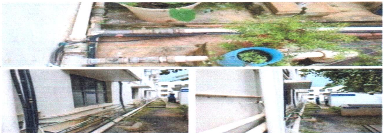
Dual water piping system installed in the campus
