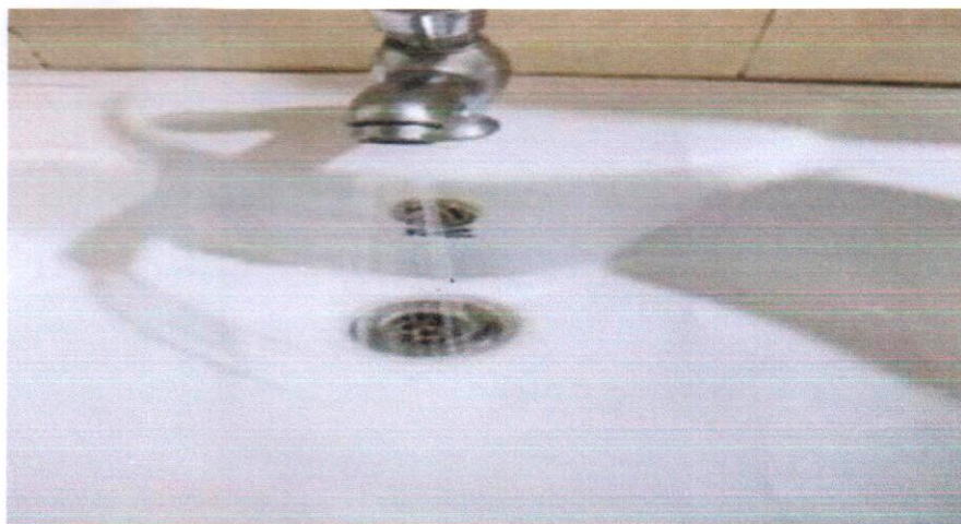
Low flow taps installed in the college
