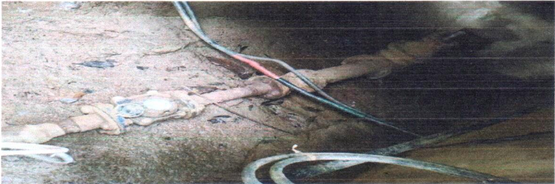
Water flow meter installed in the campus
