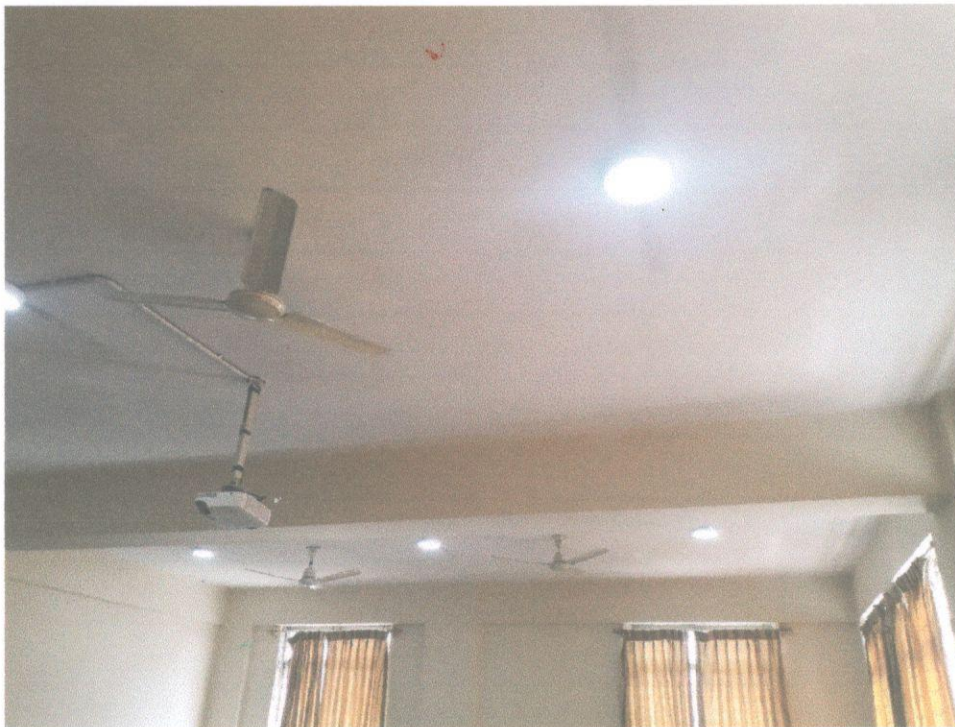
Classroom Lighted with LED bulb
