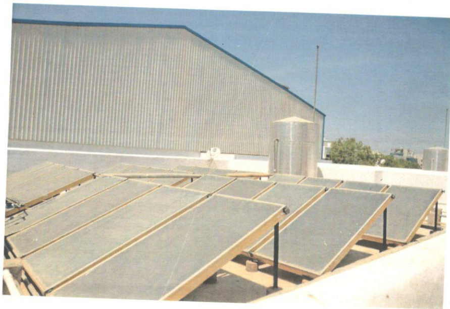
Solar panels installed at the strategic locations
