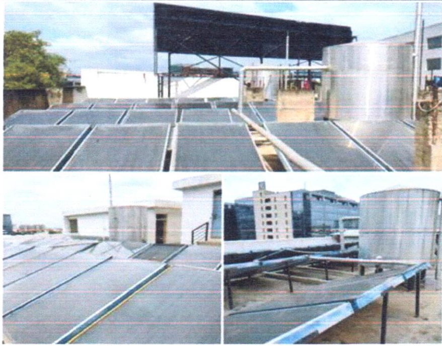
Use of Solar Water Heater
