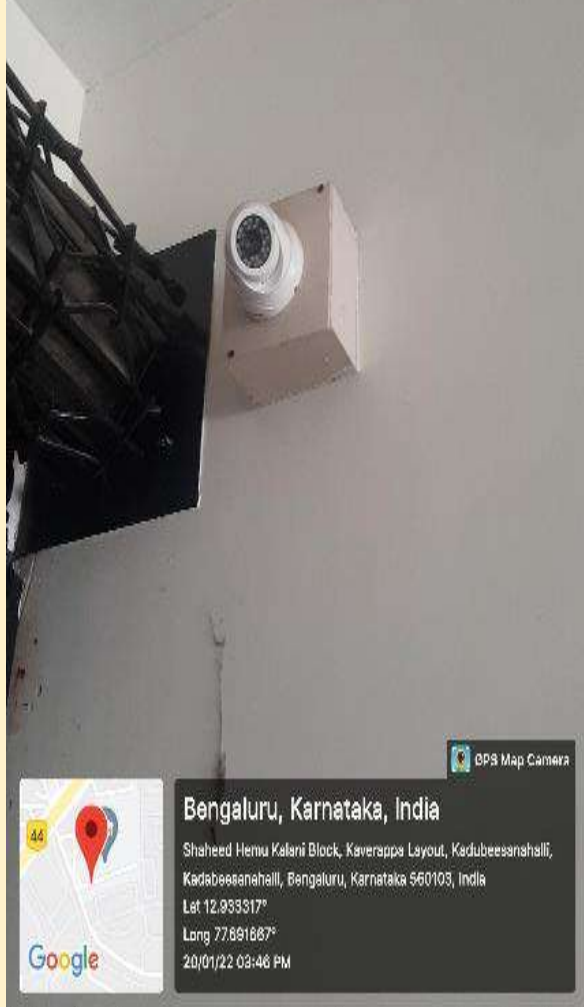
CCTV- Accounts Department
